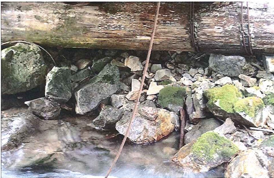
CK2463 Right Abutment Scour
